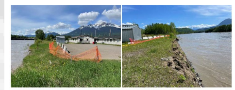
Section of road directly against the edge of the Skeena River with a 9 m near vertical drop.
